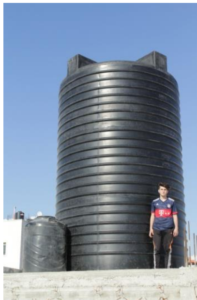
Figure 1.26: 30,000 litre water tank (Url-13).
