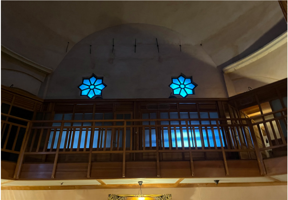
Fig. 9. (a) Women's soğukluk with stained and deteriorated marble fountain; (b) wooden changing rooms; (c) plaster deterioration above the upper-floor star windows on the cut wall (Photos: Authors, 2025)
