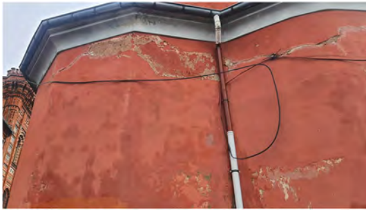
Fig. 25 Moisture problem on the east façade of Muhliotissa (Altunışık, 2024).
