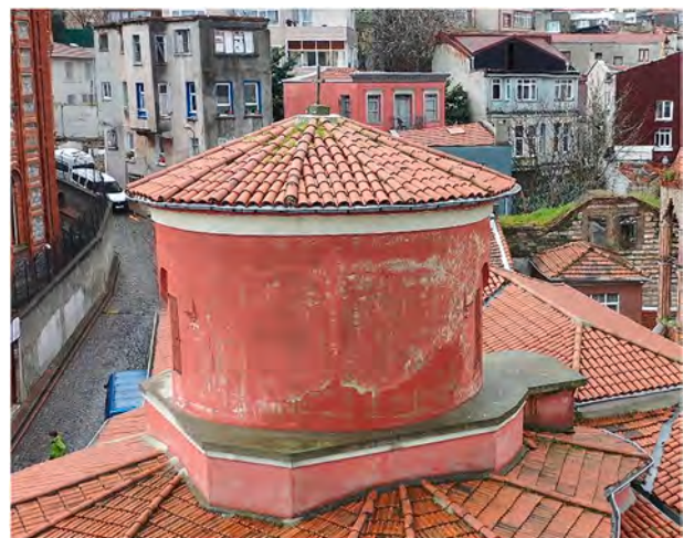
Fig. 24 Moisture problem in the main dome (Altunışık, 2024).
